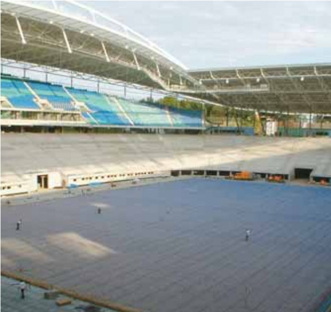
Under-soil heating system, realized by the climatherm-pipe system in Leipzig's World Cup Central Stadium
