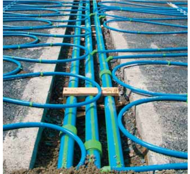
Installation of open space heating by reverse return technology
