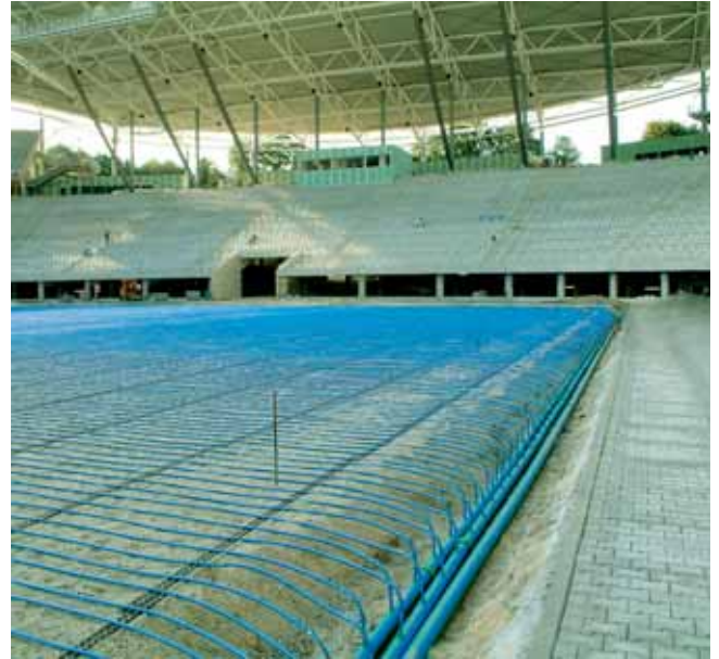
Under-soil heating system in Leipzig's World Cup Central Stadium
