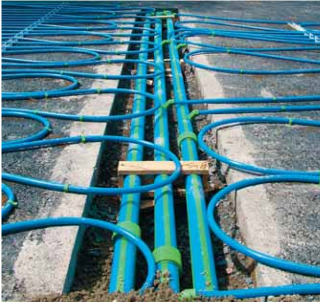
Open space heating system
