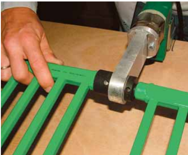
3. Push internal connection of the first grid into the (socket) heating tool and at the same time the external connection of the second grid onto the (spigot) heating tool.
