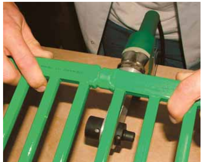
4. After the required warm-up time of 5 sec., remove the elements from the tools and immediately push together (welding depth 13 mm).
