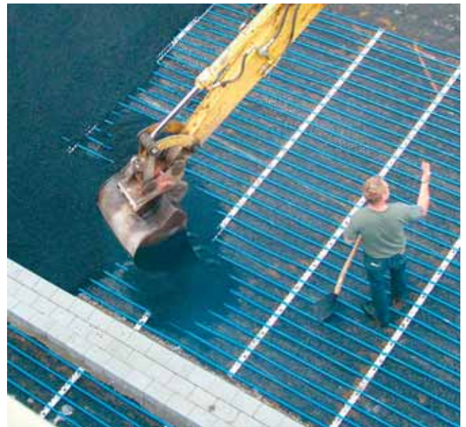
Open space heating: tar-covering of the heating system
