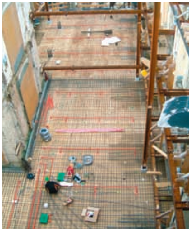
The firestop pipes are embedded in the new interim ceilings of the stripped building...
