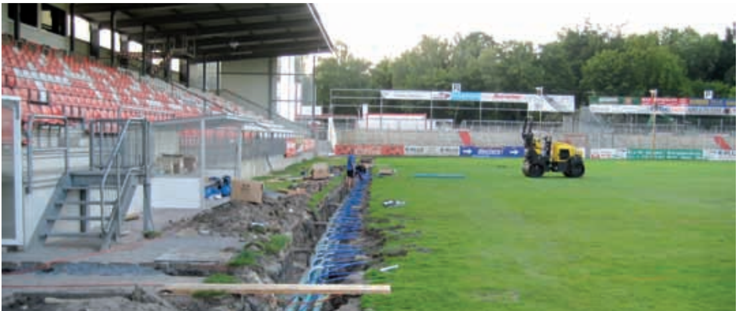
The Werse stadium in Ahlen - equipped with the climatherm-pipe system for chilled, hot fluid and various industrial applications made by aquatherm.
