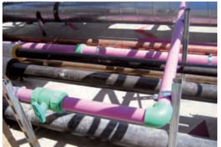
US Navy Base: Lilac pipe system for recycled water
