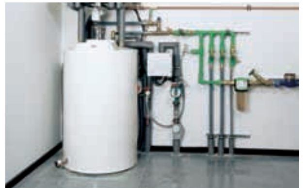
... central heating system and...
