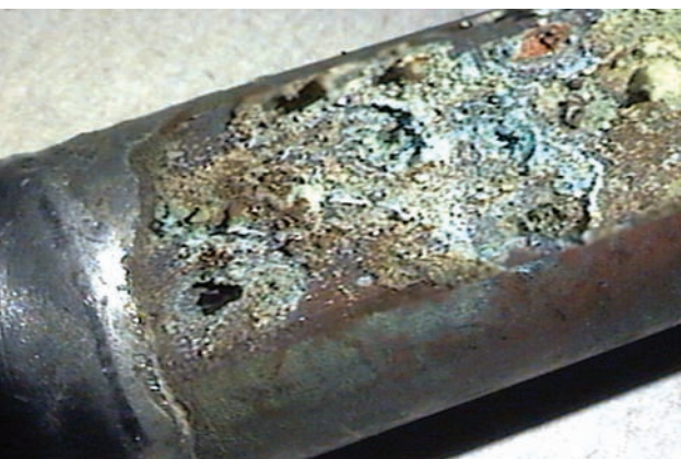
Corroding metal pipe
